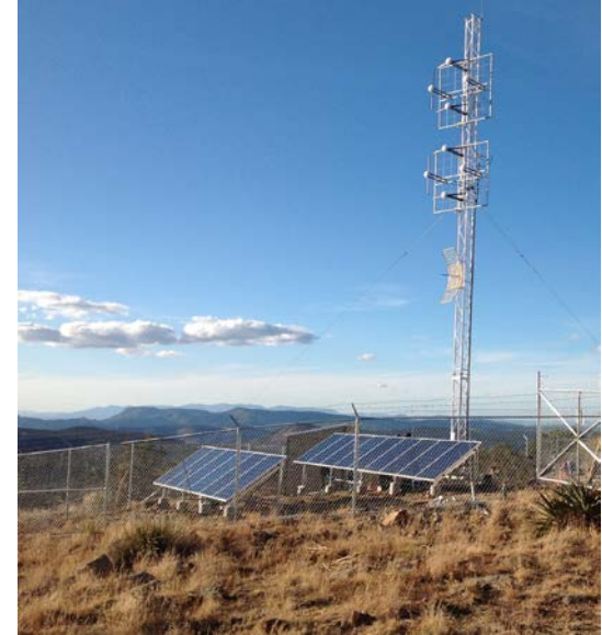
The San Carlos Apache Tribe's 10-kW solar PV system generates energy to run the tribal radio tower
