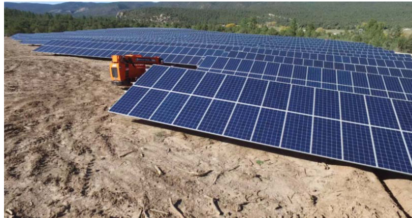
Community solar array at Picuris Pueblo
