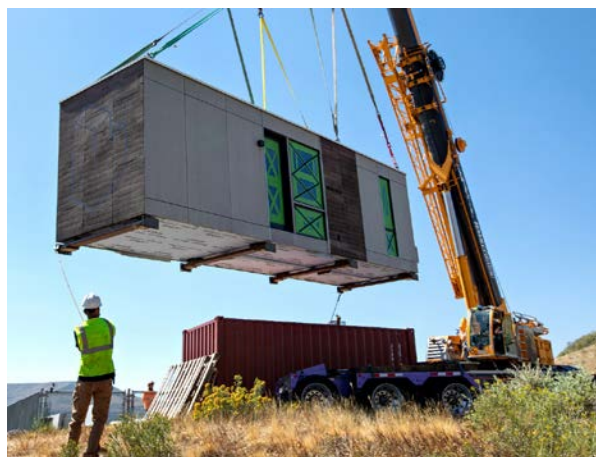
Figure 1 A modular “blok” apartment unit is craned onto site. Credit: NREL image #62503.
