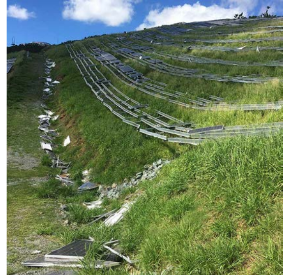
St Thomas hurricane damage. Dec. 2017. Photo by Eliza Hotchkiss/NREL
