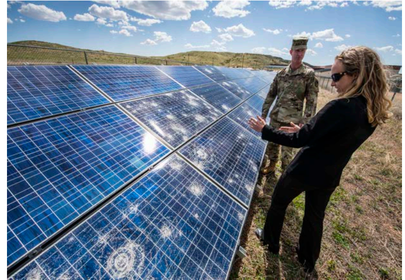
Fort Carson array 50% damage from hailstorm in May 2019. Photo by Dennis Schroeder/NREL
