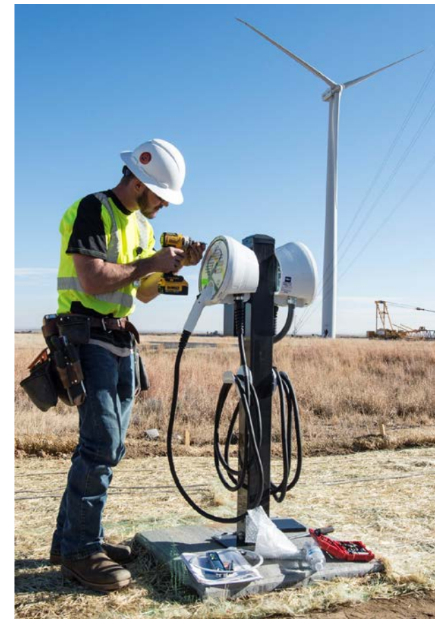
Installation of smart charging system at NREL's Flatirons Campus (Dennis Schroeder / NREL)
