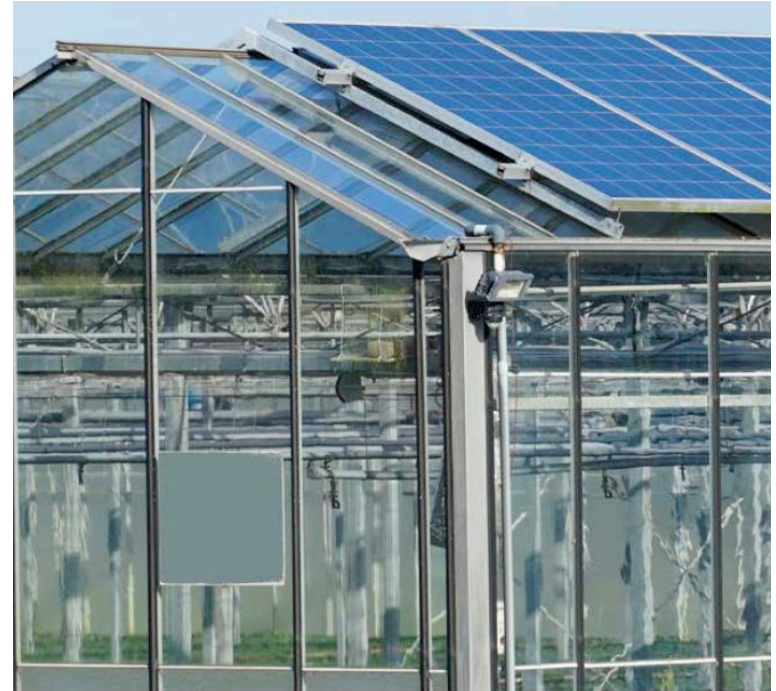
Photovoltaic solar panels installed on a greenhouse. Photo from iStock 1207270991
