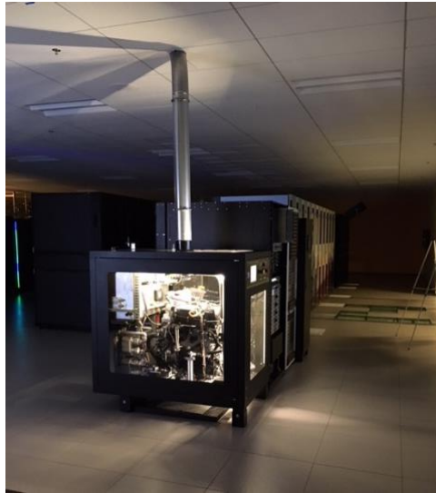
Figure 5. FC system in the HPC prior to the exhaust vent being insulated (Saur et al. 2020)
