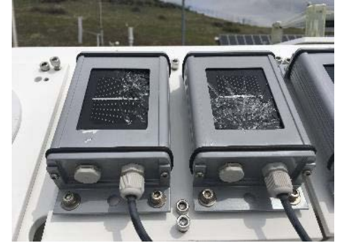
Hail Damage to Irradiance Sensor (NREL 2017)
