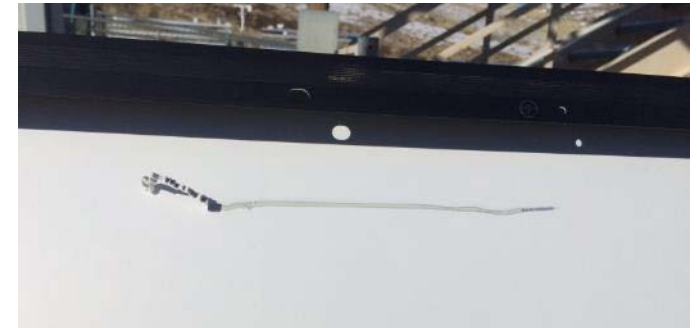
Shipping Damage – back sheet scratched during unpacking (NREL 2016)
