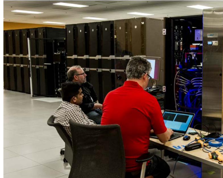
March 21, 2016 - Eric Kozubal, NREL, Harsh Patel and Daryl Lautenschlager, work on the LiquidCool Solution's "Liquid Submerged Server" at ESIF's HPC data center. (Photo by Dennis Schroeder / NREL)
