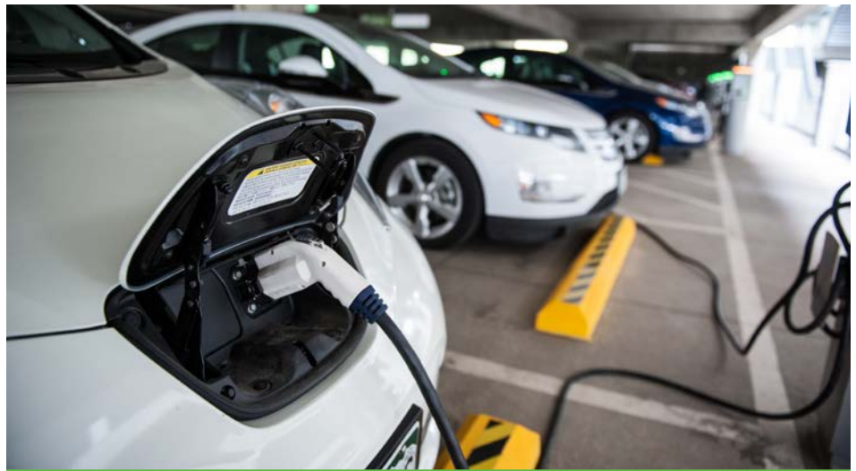
Figure 1. Workplace charging may be co-located with fleet EVSE or installed simultaneously to achieve cost savings. Here, an electric vehicle is plugged into a charging station in the NREL parking garage. Photo by Dennis Schroeder, NREL 26669.
