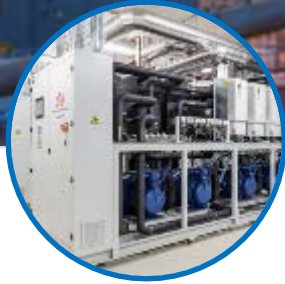
High Temperature Heat Pump (HTHP) System for District Heating
