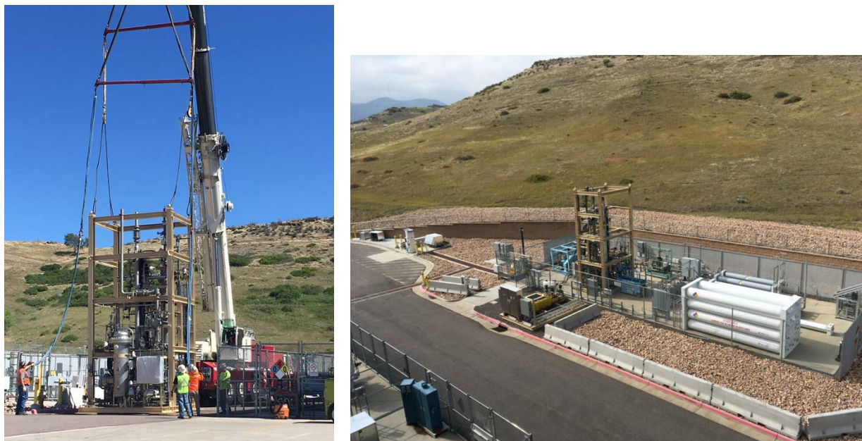
Figure 3. Installation (left) and fully assembled operation (right) of the SoCalGas bioreactor and supporting infrastructure at the ESIF. Photos by NREL
