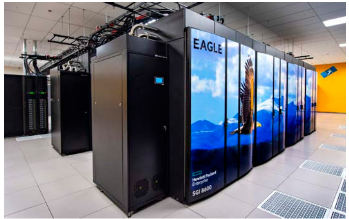
NREL's high-performance computing system, Eagle. Photo by Dennis Schroeder, NREL 53840
