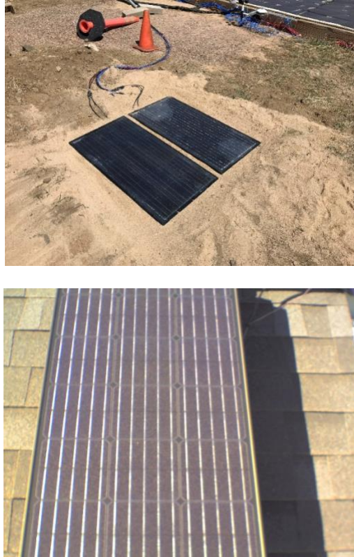
Fig. 3. Triple composite PV modules installed on ground as pavers (left) and a non-triple composite PV module mounted on an asphalt shingle sloped roof surface (right). Corresponding to their data logger channel assignment, the left paver module is referred to as M102 and the right paver module is referred to as M104. More delamination is evident for M104 on the right.
