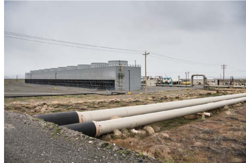
Blue Mountain Geothermal Plant , Nevada Geothermal Power (NGP), Humboldt County, Nevada. Waste water pond. (Photo by DENNIS SCHROEDER / NREL)
