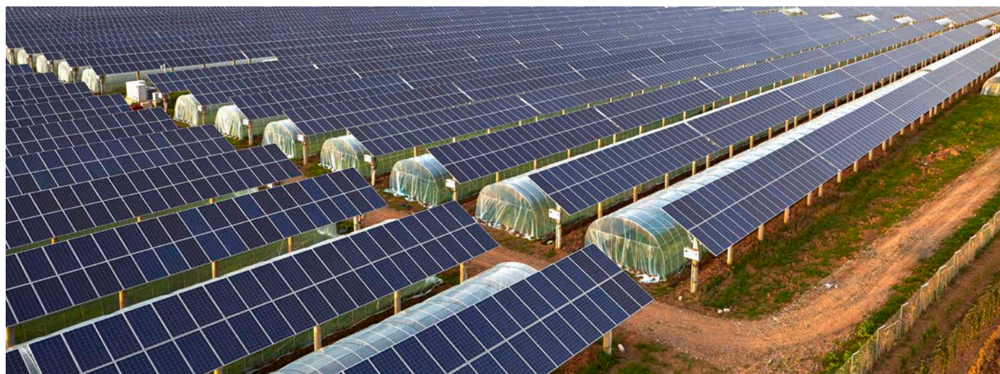
Solar photovoltaic panel built on the roof of aerial vegetable greenhouse. Photo from iStock 1131751289
