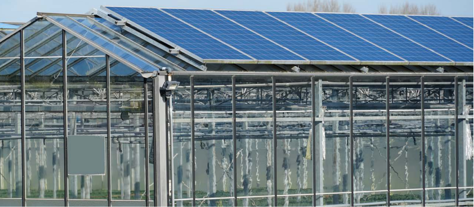
Photovoltaic solar panels installed on a greenhouse. Photo from iStock 1207270991
