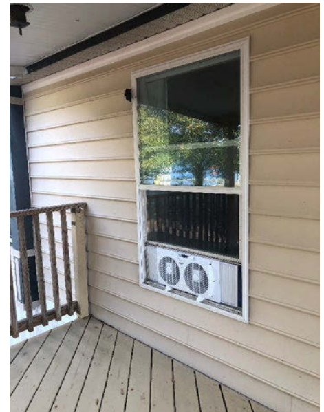
Figure 4. Window fan installed in the main zone providing outdoor air into the home. This pressurizes the main zone, resulting in a lesser pressure in the closed-off isolation zone with reference to the main zone, which helps with containment. Photo courtesy of FSEC
