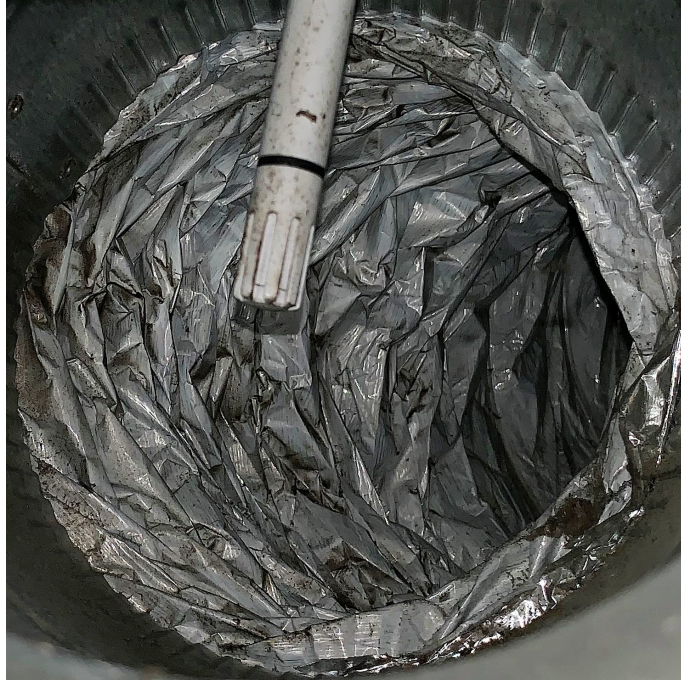
Figure 27. Photo of inside of X_1 duct from test home 3 (representative of the X_1 duct in other homes)
