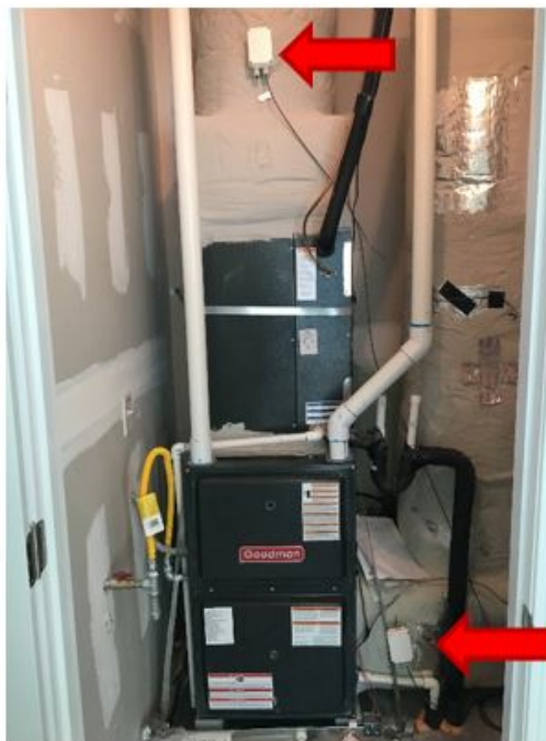
Figure 11. T/RH probes in the supply and return plenums of the AHU
