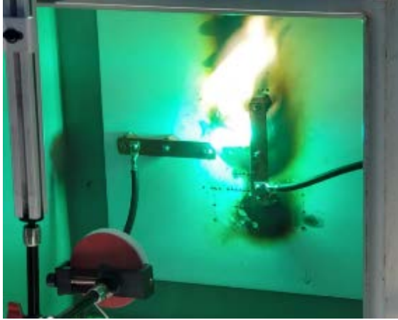
Fig. 16 – Flat Tee Bus arc test showing arc elongation between bus bars (NREL)
