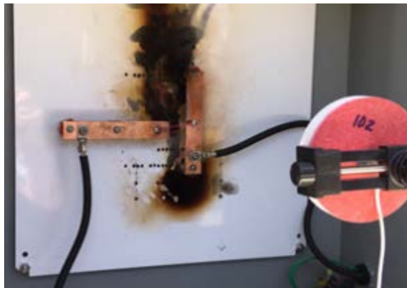
Fig. 9 - Flat Tee Bus Bar Configuration as tested (NREL)
