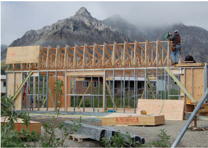
Anaktuvuk Pass, Alaska: A local crew builds an energy-efficient home in 2008 in the Inupiaq village of Anaktuvuk Pass. Designed by the CCHRC, the home blends innovative technologies such as a foam raft foundation and super-insulated envelope with traditional techniques like earth-berming to stay warm.
