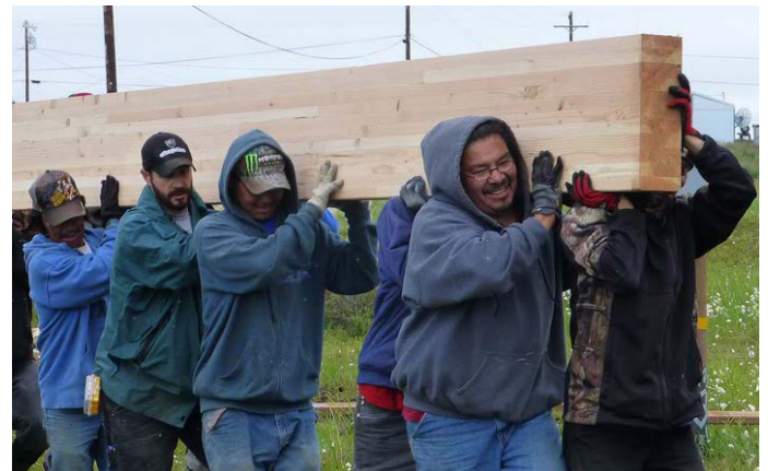
Atmautluak, Alaska: CCHRC trained a Yup'ik crew to build two super-energy-efficient homes in this southwest Alaska village in 2013. With no heavy equipment or trained carpenters in the village, the home was designed to be lightweight and simple to assemble. The adjustable foundation can move with the highly active ground.
