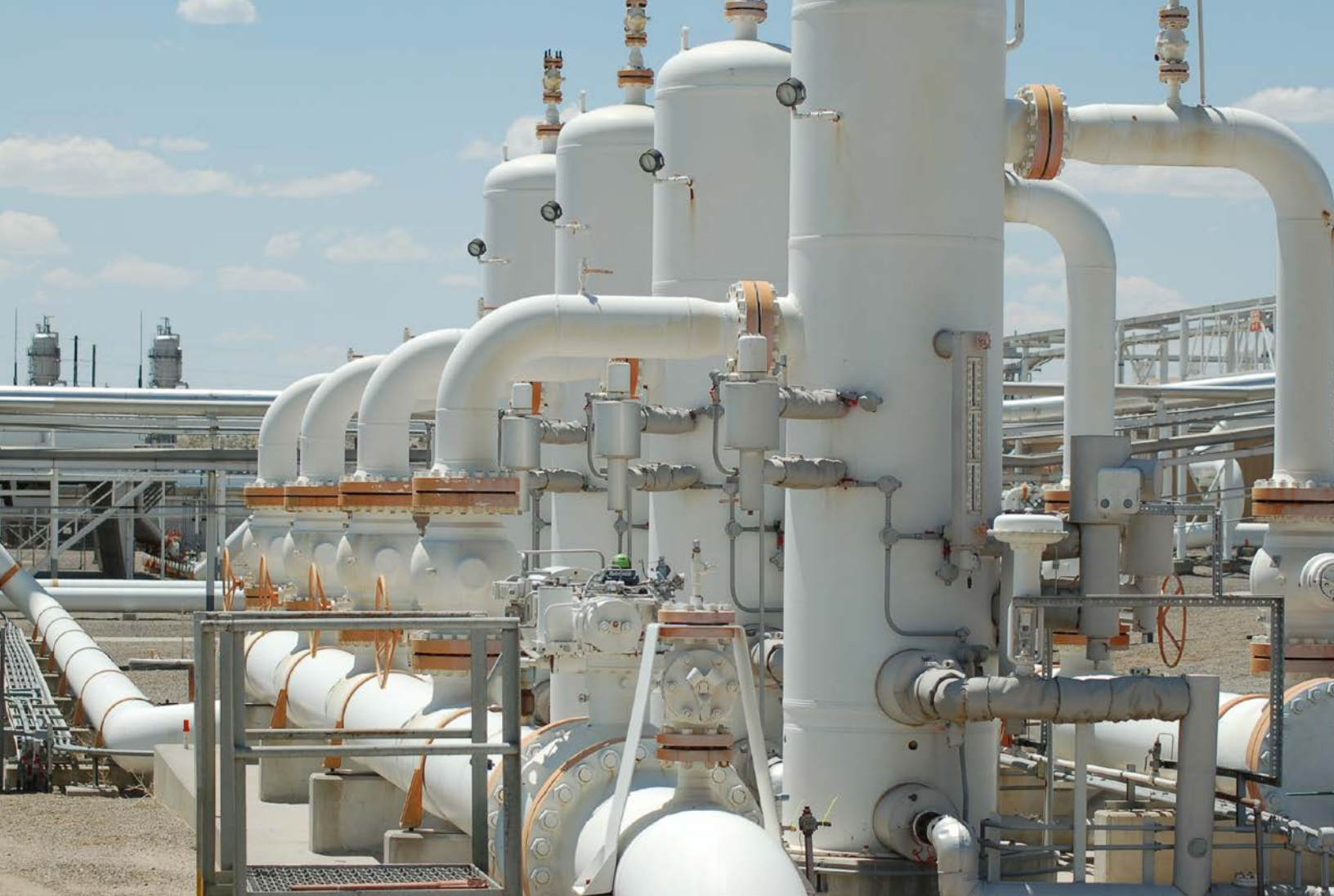
Streamlined coordination between the natural gas and electric sectors can alleviate many challenges natural gas operators face today with the evolving U.S. power grid. Photo courtesy of Kinder Morgan
