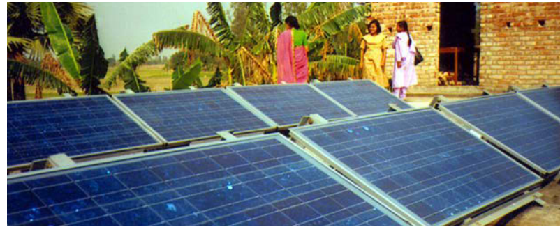
Solar modules installed on the roof of the Satyanarayanpur Health Center in West Bengal, India. Photo from West Bengal Renewable Energy Development, NREL 08904
