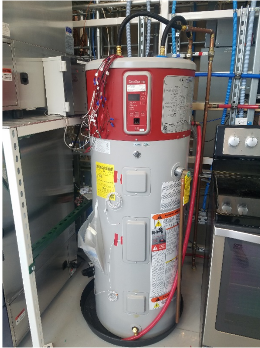
Figure 7. GE HPWH with external controls
