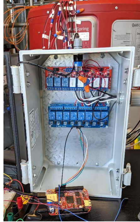
Figure 8. Control board and relays for external controls
