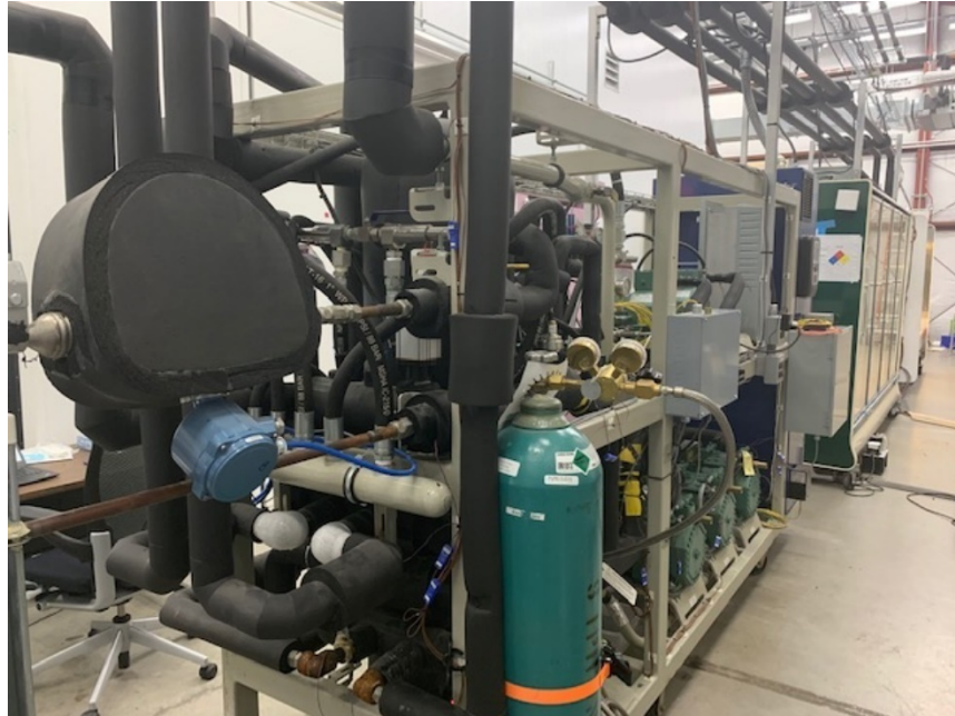
Figure 6. Commercial refrigeration system
