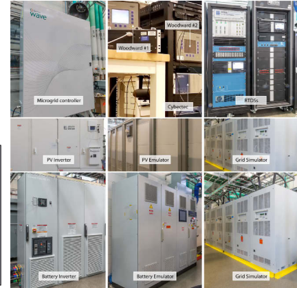
Pictures of physical equipment
