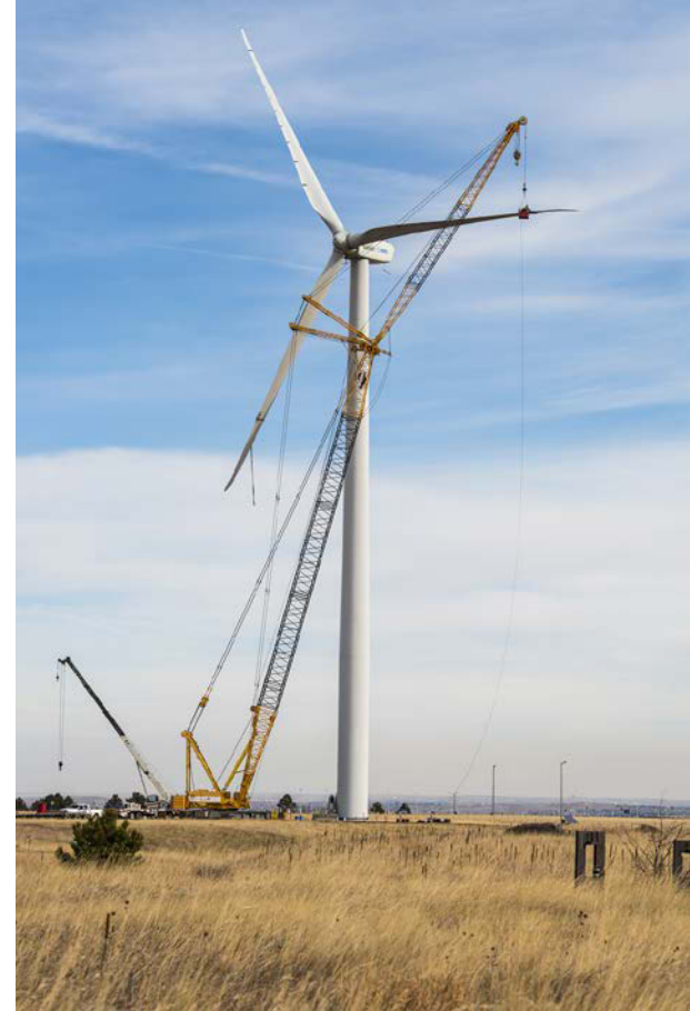
Photo by Dennis Schroeder, NREL #49389
