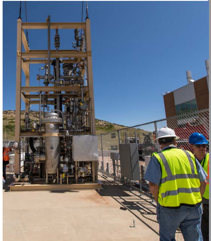
Crews work to install the first U.S. Power-to-Gas system outside the ESIF. Southern California Gas partnered with NREL on the project, which takes excess electricity and converts it to hydrogen which can be used, stored or combined with carbon dioxide to produce renewable natural gas. Photo by Werner Slocum, NREL 47268
