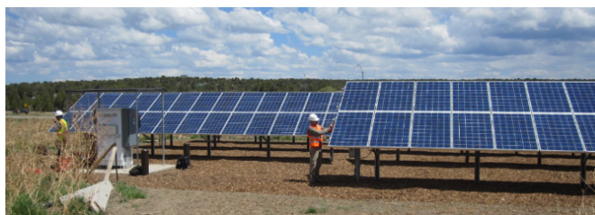
Fig. 9 PV array and inverter at Mesa Verde National Park
