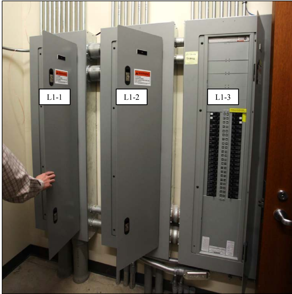
Figure 23. Location of Panel L1-3 within the site electrical room at Havana Gardens
