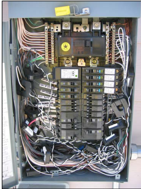
Figure 2. Residential electrical panel with CTs installed on all breakers
