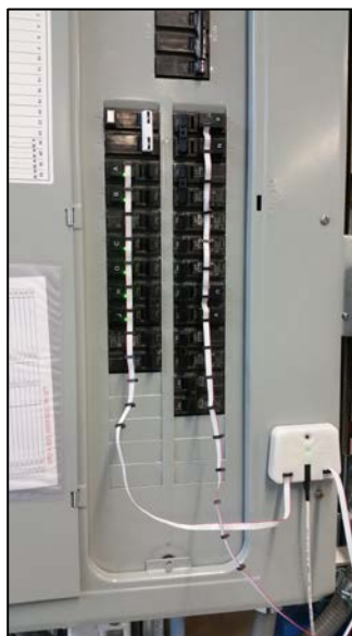
Figure ES2. The Whisker Labs meters installed on the front of breakers in an electrical panel.
