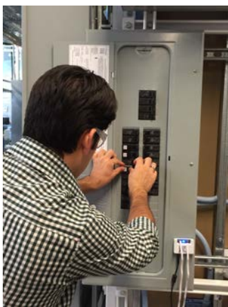
Figure 9. Step 1 – Use stencil as a guide to position the sensor on the breaker
