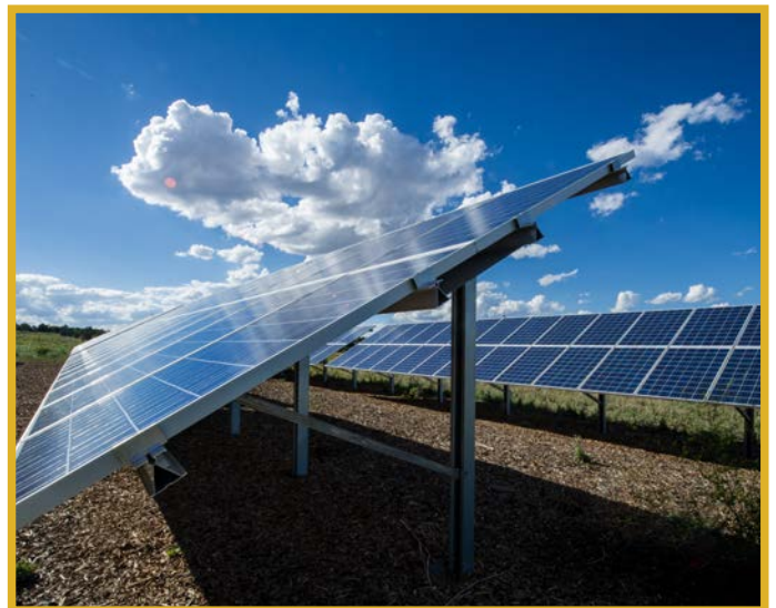
Photo by Dennis Schroeder, NREL 26961
