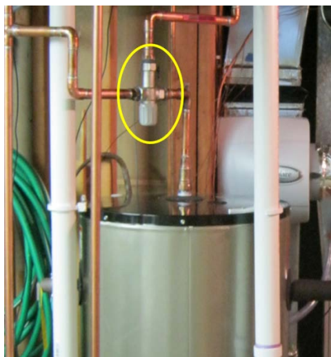
Figure 7. DHW mixing valve
