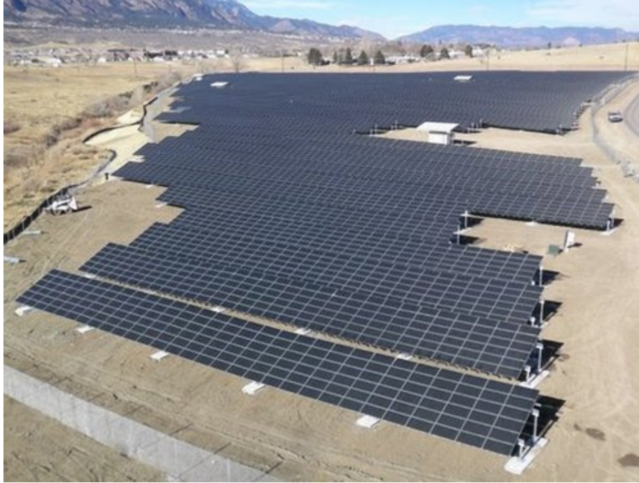
Figure 14. PV system with fixed tilt
