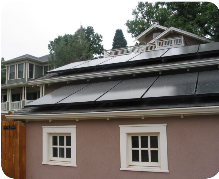
Solar panels placed on an accessory structure not visible from the public right of way should still follow the slope of the roof and have a low profile. Photo courtesy of Dan Corson
