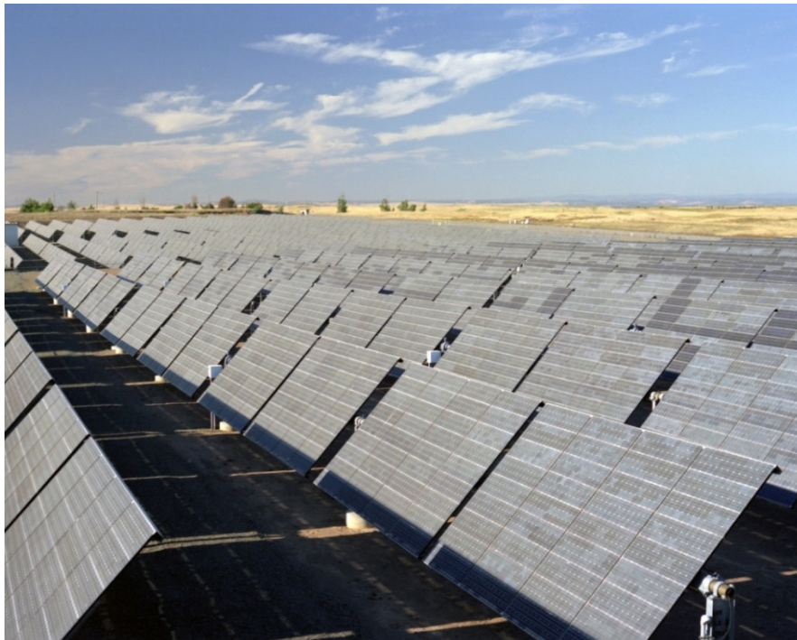
Figure 15. PV system with single-axis trackers
