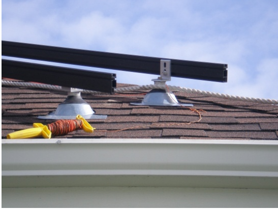
Source: NREL PIX 21403
