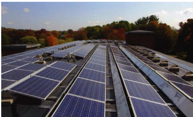
Solar panels installed on the flat roof.
