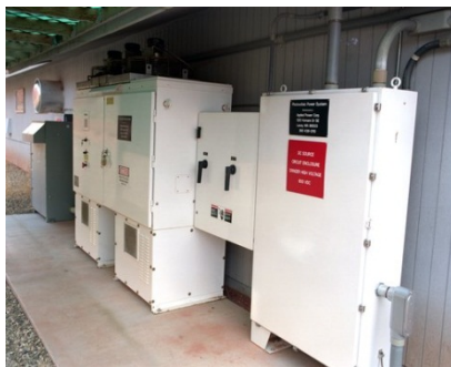
Source: NREL PIX 07985
