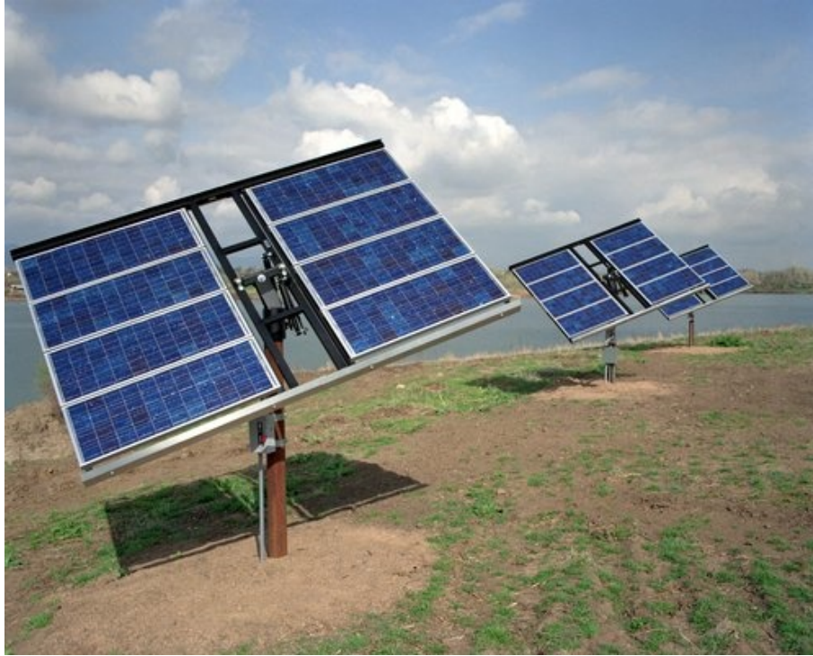
Figure 16. PV system with dual-axis trackers
