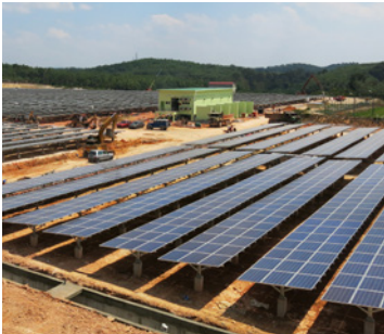
Amcorp Gemas 10.25 MW solar power plant in Gemas, Negeri Sembilan, Malaysia. Photo courtesy of Amcorp
