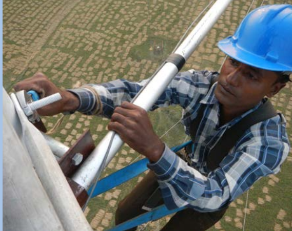
Lead tower construction manager for Sitakunda installs instrumentation on 80 meter Meteorological “Met” Tower used to measure the wind resource in Bangladesh.
