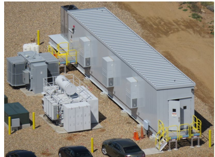
Controllable grid interface. Photo by Mark McDade, NREL 29069
