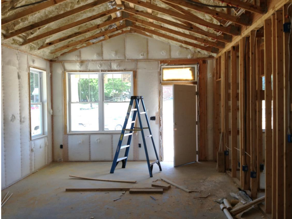
Figure 20. Netted Spider insulation
