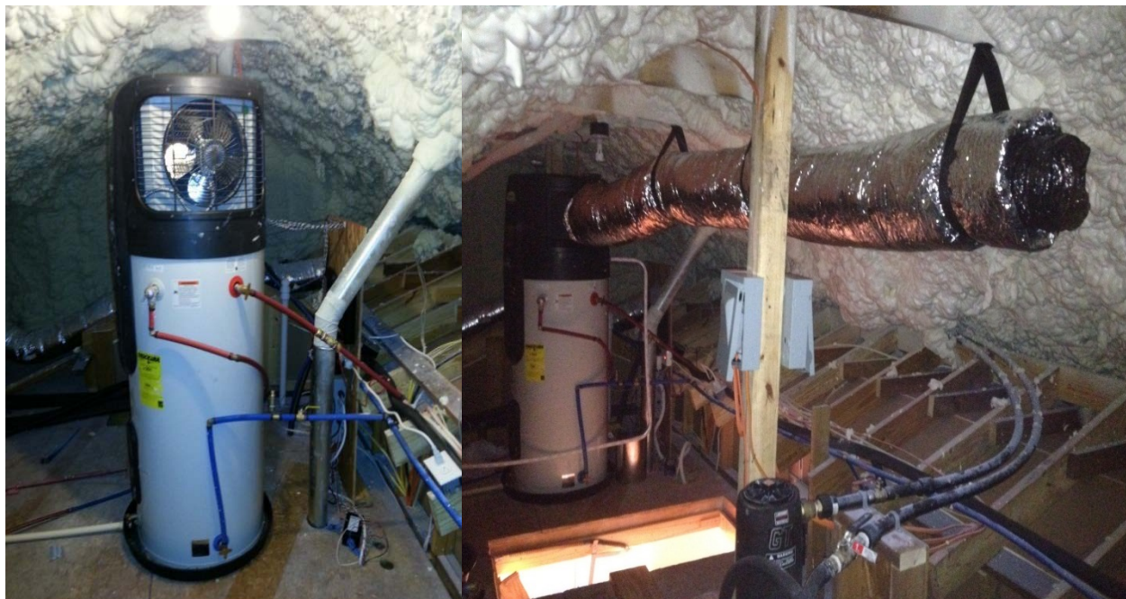
Figure 27. Savannah Gardens Lot 207 HPWH in the encapsulated attic before the exhaust duct was installed (left) and after the exhaust duct was installed (right)
