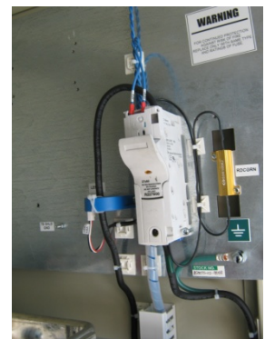
Figure 1. Typical ground fault fuse holder
