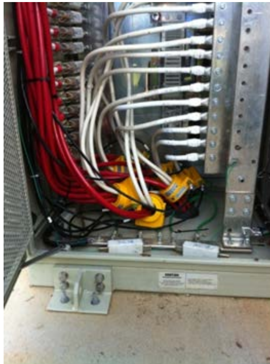
Figure 7. Multiple current transducers in PV output circuit combiner
