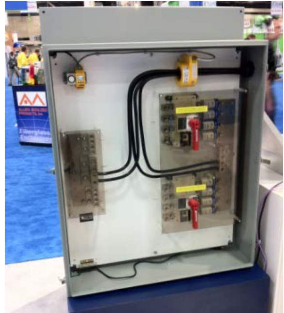
Figure 9. PV output circuit combiner equipped with residual current monitor
