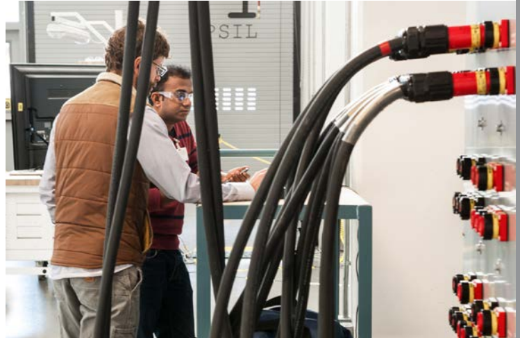
Solectria is leveraging the unique capabilities of the ESIF to test its advanced inverter technology. Photo by Dennis Schroeder, NREL 30499
