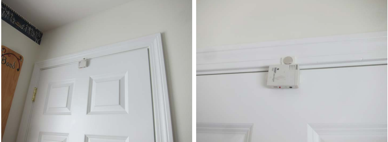
Figure 16. Door open/closed sensors
