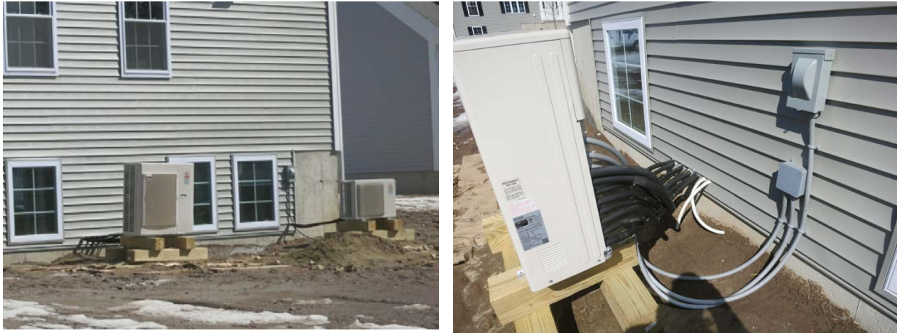
Figure 9. 3:1 multisplit DHP (Mitsubishi MXZ series) installed at Easthampton
