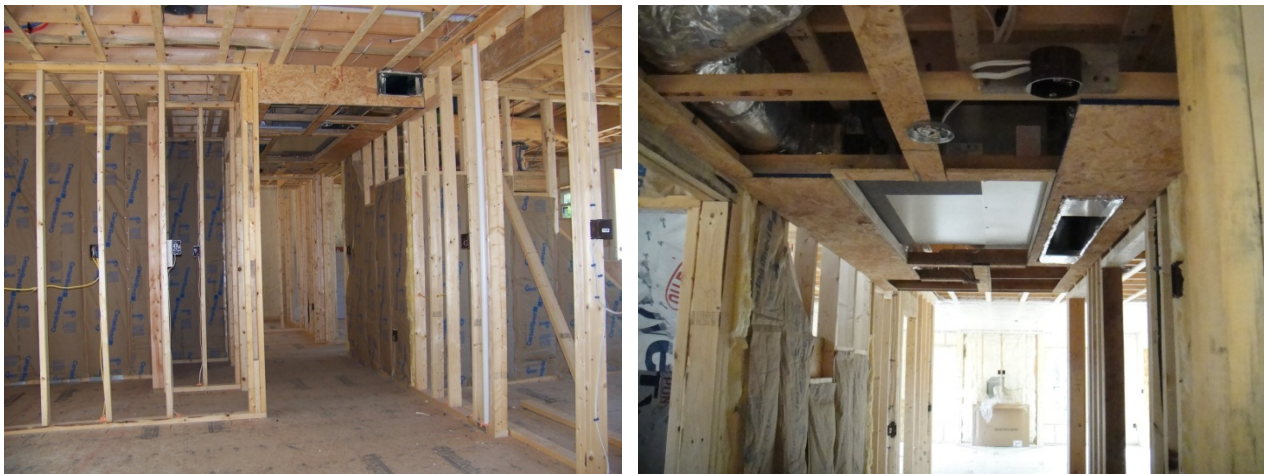
Figure 10. Ducted air handler MSHP indoor unit, at Transformations’ Townsend development
