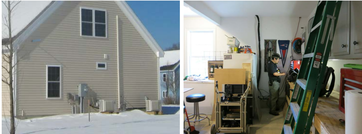
Figure 79. Retrofitted unit and line set for second-floor MSHP on exterior (L), and in garage (R)
