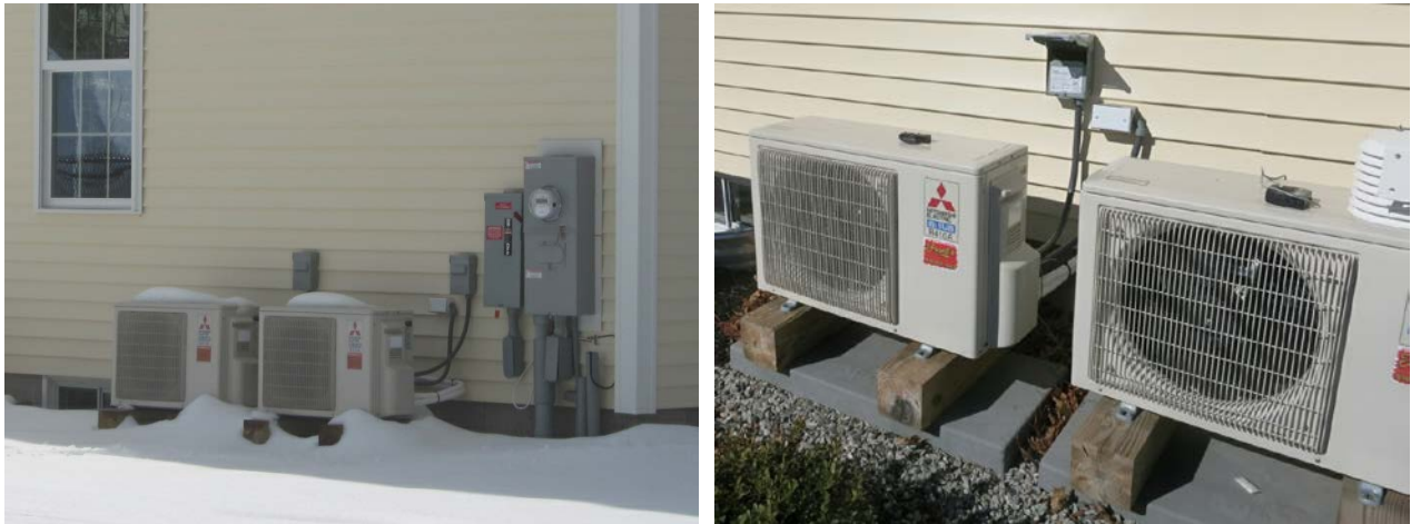
Figure 34. Outdoor units raised on wood block risers
