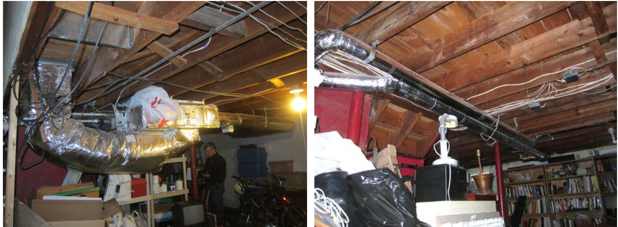
Figure 11. Ducted air handler MSHP indoor unit, with excessively long/restrictive ductwork
