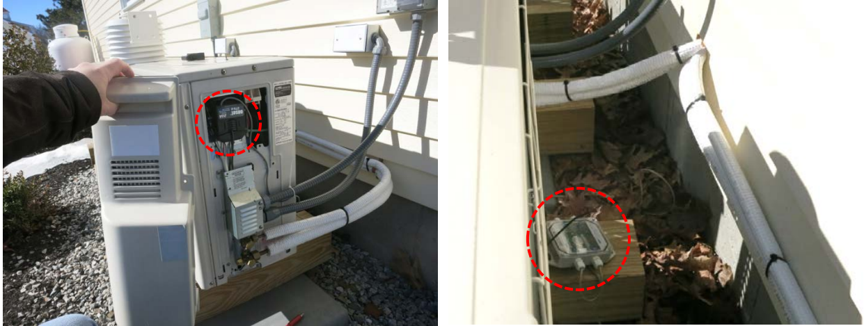
Figure 18. MSHP electrical power monitoring at outdoor unit
