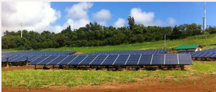
1.2-MW PV array on Kauaʻi. Photo by Jamie L. Keller, NREL 21774
