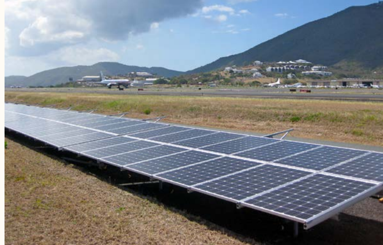
A 448-kW PV system installed at the Cyril E. King Airport on St. Thomas in April 2011. Photo by Adam Warren, NREL 18953
