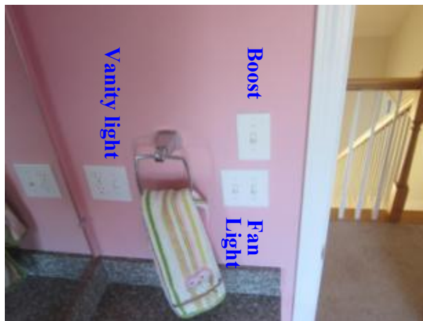
Figure 48. Light, fan, and wall switches
