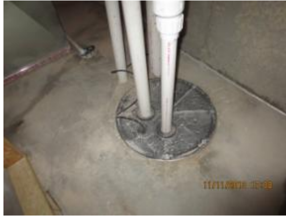
Figure 19. Airtight sump cover and air sealed radon pipes at Plan 601
