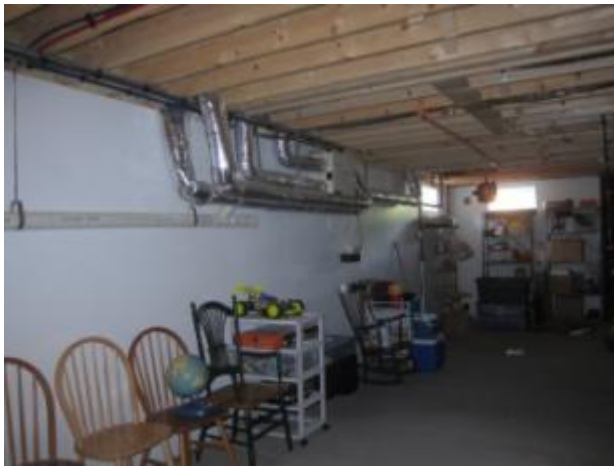
Figure 44. Fantech SH704 HRV in basement
