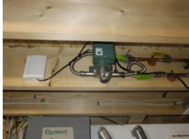
Figure 15. Location of Taco D'Mand recirculation pump
