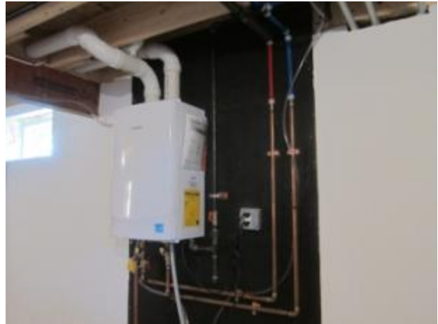
Figure 36. Navien NR-180 (LP) unit installed in basement
