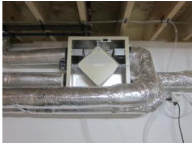
Figure 45. Fantech SH704 HRV in basement
