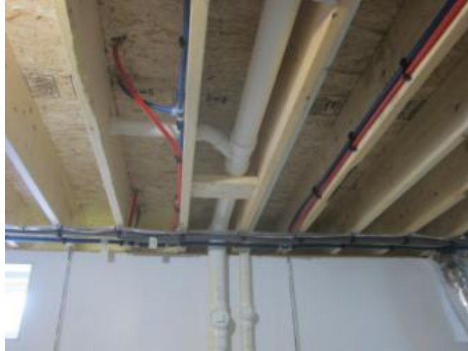
Figure 9. Hot and cold ½-in. branches from ¾-in. insulated trunk
