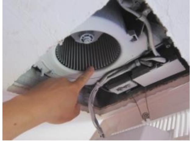
Figure 47. No flow at Panasonic fan with switch off
