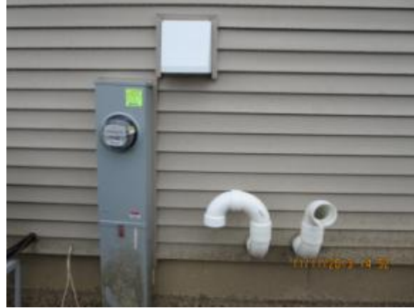
Figure 31. First-floor bath exhaust termination
