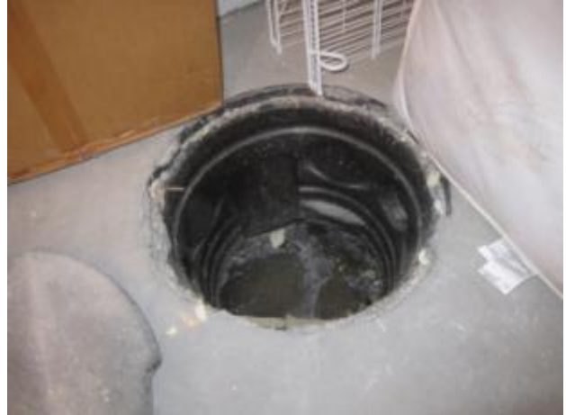
Figure 23. Standing water in sump, Lot 6
