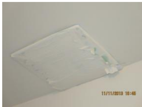
Figure 18, Garage fan at K. Hovnanian Plan 601 (grille is covered for protection during construction)
