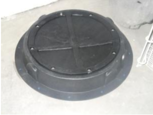
Figure 26. Sump pit retrofit cover, Lot 6
