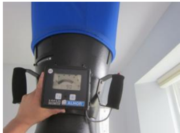
Figure 43. Flow measurement at bathroom exhaust
