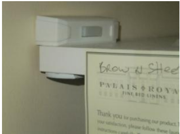
Figure 17. Remote button in laundry room
