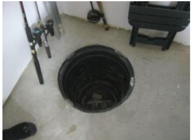
Figure 25. Dry conditions in sump, Lot 7
