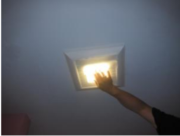
Figure 46. Testing bathroom exhaust fan for flow
