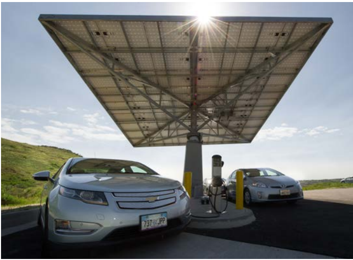
Plug-in hybrid EVs charge at the rapid charging system powered by a solar canopy at the Vehicle Testing and Integration Facility at the National Renewable Energy Laboratory.
