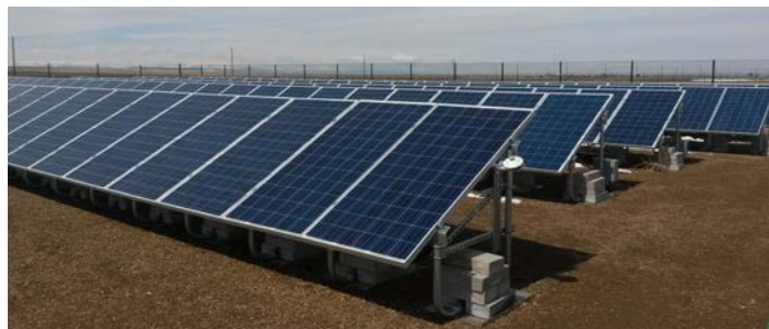
Fig. 7: Maxim installation at the Colorado RTC site
