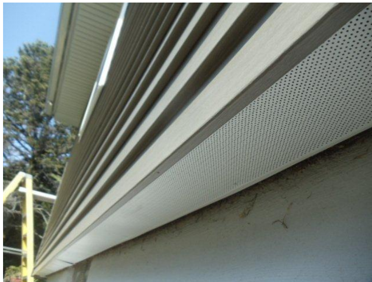
Figure 26. Insect guard and ventilation at the bottom of the wall system
