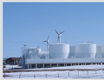
Alaska Village Electric Cooperative installed three 100-kW Northern Power Systems turbines in November 2006 as part of a wind-diesel hybrid system. Two of three wind turbines can be seen in this photo over the bulk fuel tanks of the Kasiglutik Power System. Photo by Ian Baring-Gould, NREL 16097
