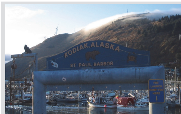
Three of six GE 1.5-MW wind turbines installed on a ridge above Kodiak, Alaska, as part of a hydro-wind-diesel power system that provides more than 95% of the community's electrical energy from renewable energy sources. Photo by Ian Baring-Gould, NREL 29181
