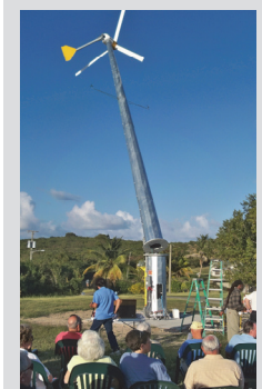
The tower of the wind turbine installed at St. Croix Reformed Church and Kingshill School can be hydraulically raised or lowered depending on weather conditions. Photo from Don Buchanan, NREL 20186
