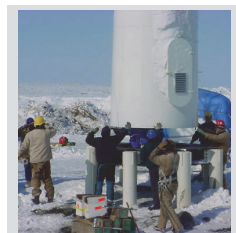
Photo from Northern Power Systems, NREL 13853
