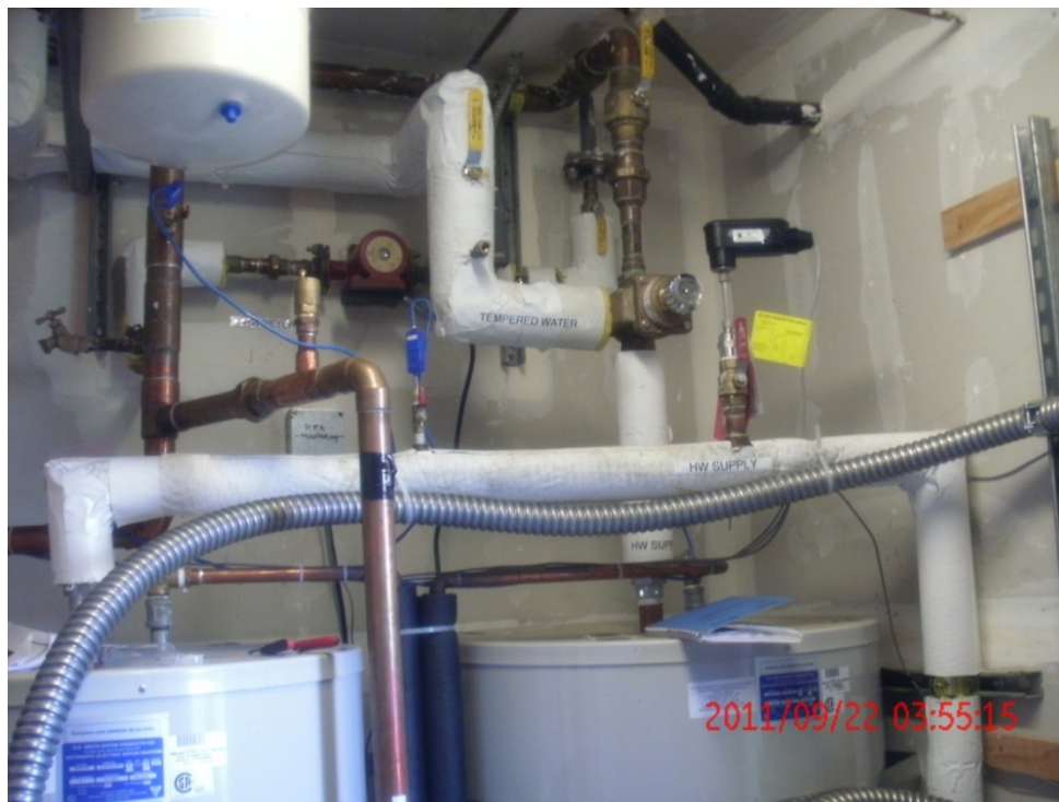
Figure 5. 120-gal electric resistance storage tanks with piping and monitoring sensors
