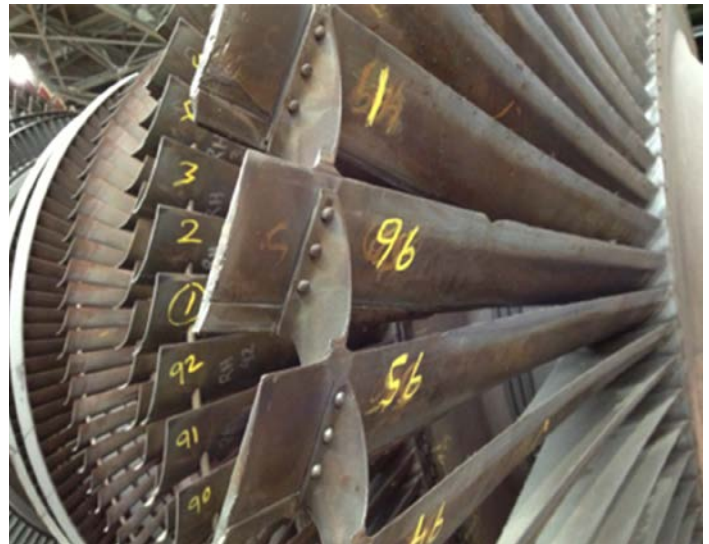
Photo by Debra Lew, NREL
