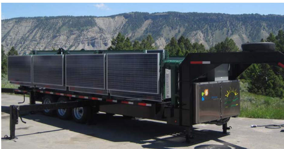
Figure 2. Mobile PV system shown stowed on the trailer upon delivery to Yellowstone National Park. Photo: Jim Evanoff
