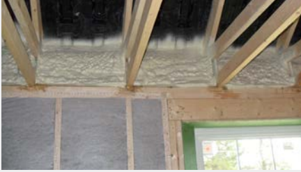
Ten-and-a-half inches of dense-pack cellulose in double 2×4 walls, raised heel trusses, and foamed-in plastic rafter vent baffles.
