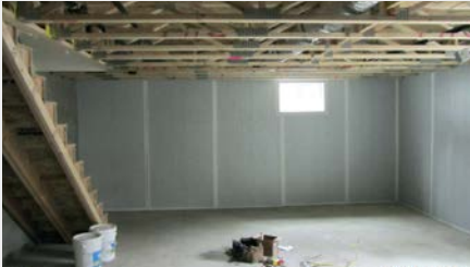
Exposed polyisocyanurate insulation panels in basement provide R-13 insulation and a finished appearance. All floor framing is open-web trusses to accommodate mechanicals.
