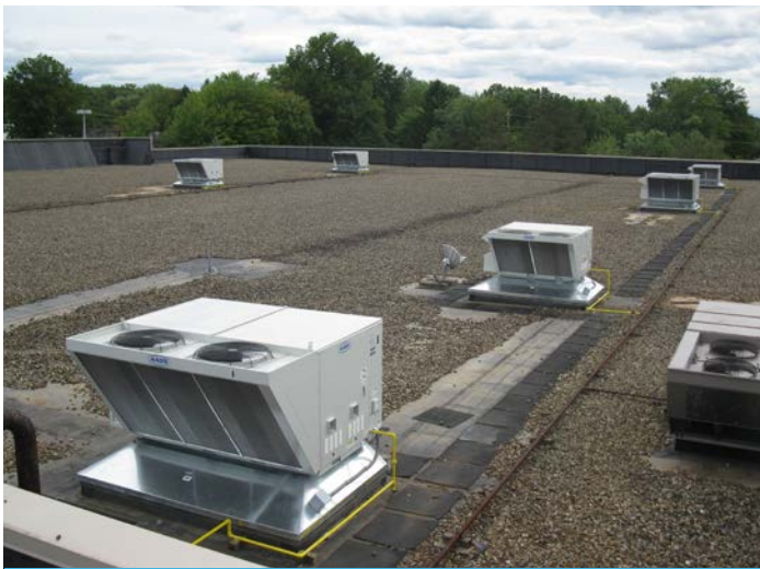
Kohl's replaced the store's aging RTUs with these new high efficiency units featuring variable speed supply fans and modulating compressors. Photo Courtesy of Kohl's
