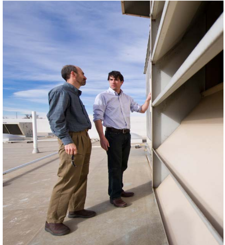
NREL researchers examine HVAC units on the roof of a Target store. Photo by Dennis Schroeder, NREL 19507
